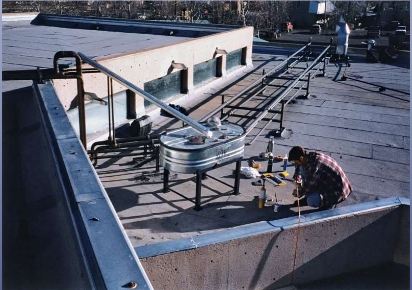
Desert Fountain. Rainwater harvesting system.
